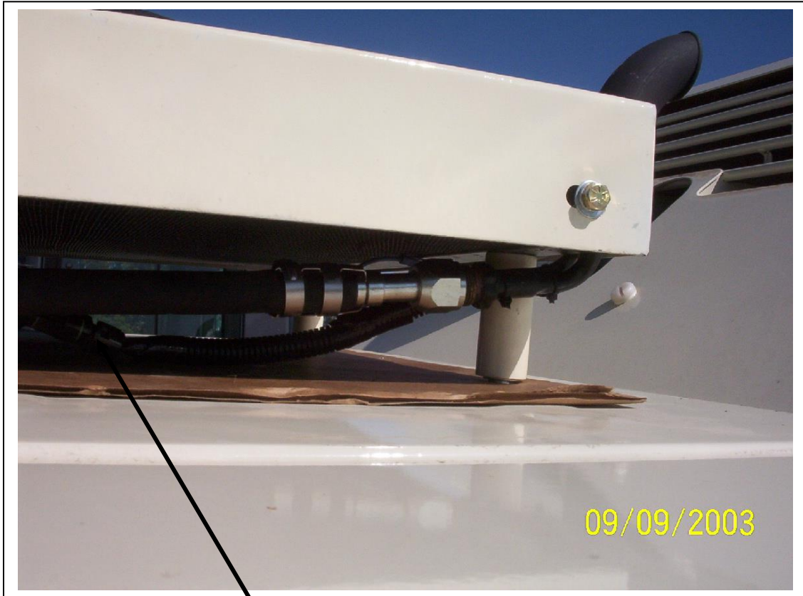
Wire connection at condenser for condenser fan power
